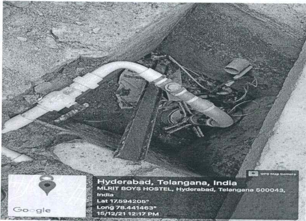
Fig:2.3: Bore well Near Boys Hostel
